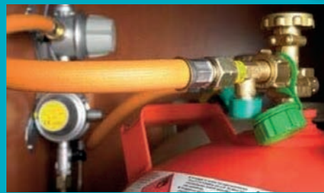
Gas Safety Check
